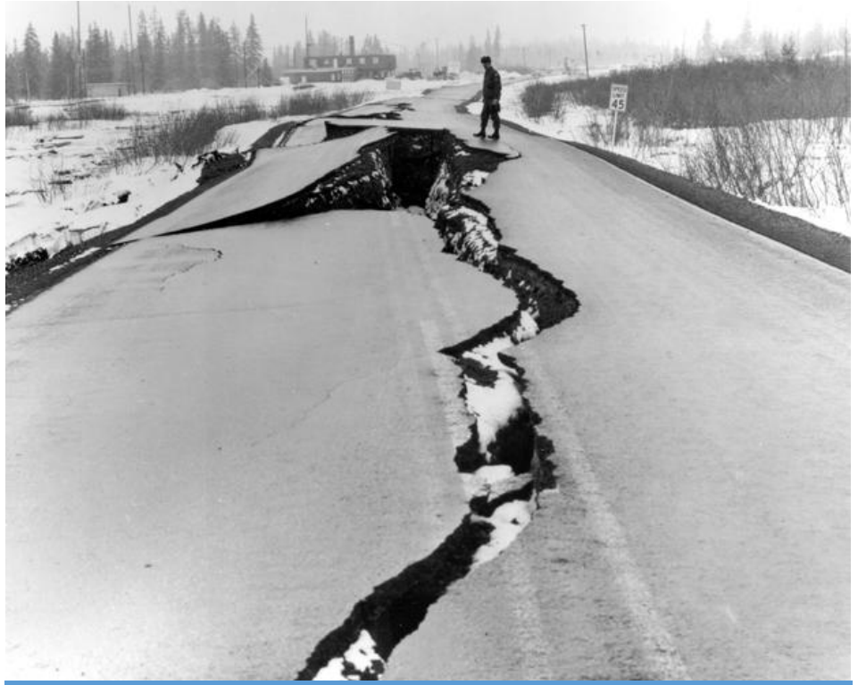
Cracks along Seward Highway, near Turnagain
